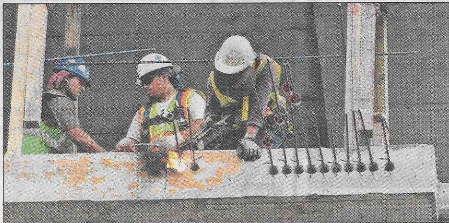
A crew works on concrete flooring in the $50 million Greenbridge project Thursday. Some say Greenbridge developers had planned to hire locally.
